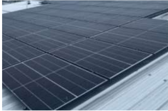
Figure 1: The photographic view of the roof type solar power plant
